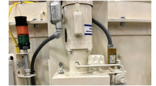
Mixer transmission lube station with pump and filter
