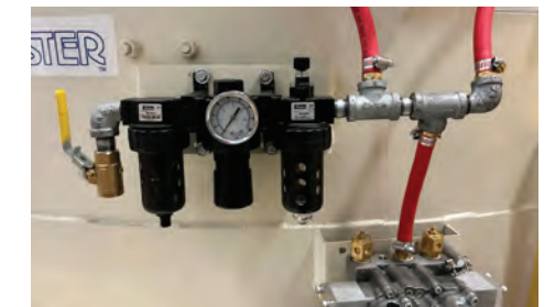
Air filter/regulator/lubricator for all pneumatic cylinders and valves supplied
