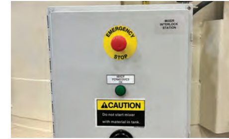
Mixer interlock station with E-Stop, warning horn & strobe and hour meter
